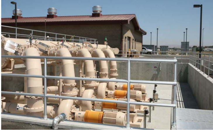
Figure 2-9. City Water Reclamation Facility
