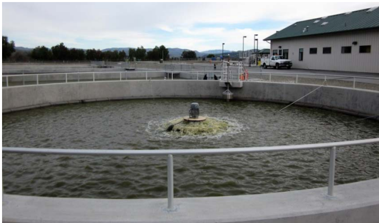
Figure 2-10. SSCWD Ridgemark Wastewater Treatment Plant
