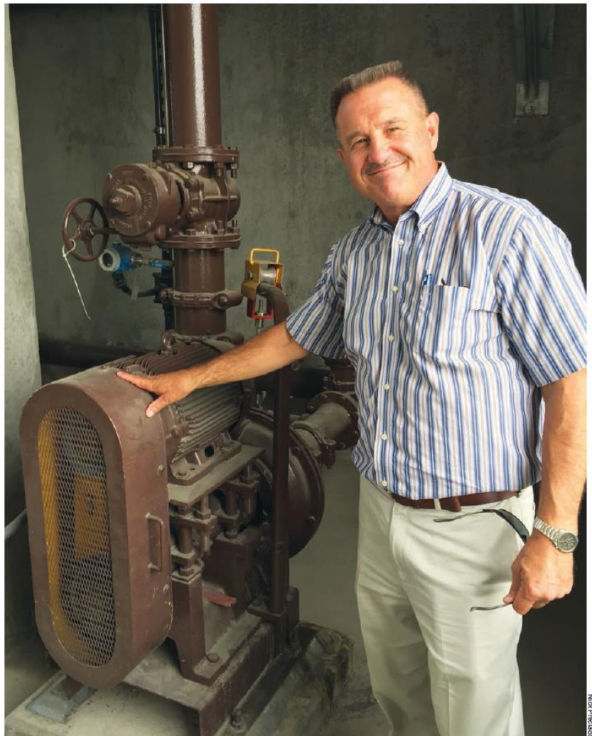
COOL ENGINEERING Sunnyslope County Water District General Manager Don Ridenhour stands with equipment inside the new West Hills Water Treatment Plant, expected to go into operation at the end of the month.
