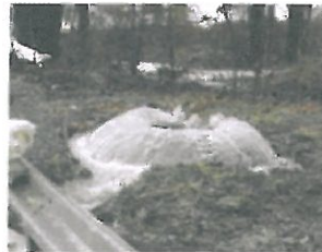
Sewer Manhole Overflow
